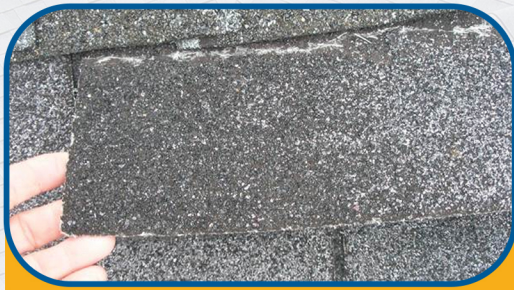
Balding Worn Down Shingles
